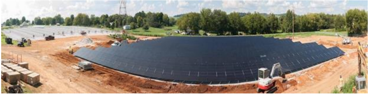
Photo: Appalachian Electric Cooperative's 1.37MW community solar array being installed by Solar Alliance in 2016.
