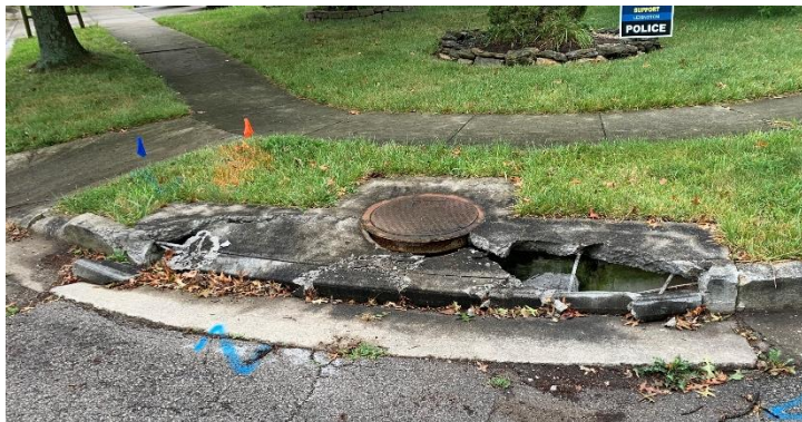
Completely Broken Inlets
