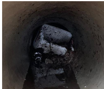
Coolers blocking Storm Pipes
