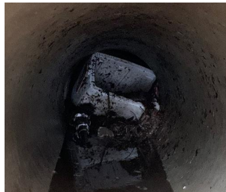
Coolers blocking Storm Pipes
