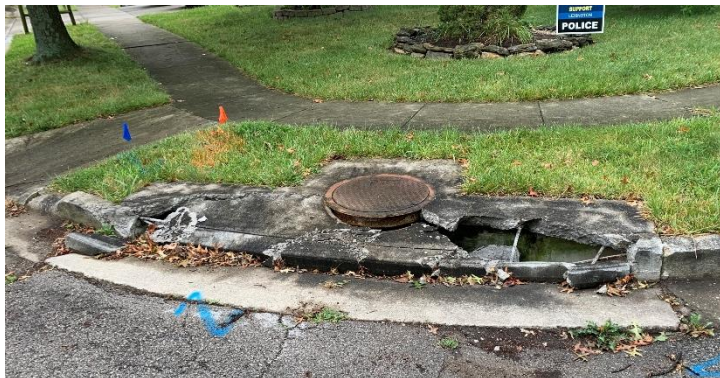
Completely Broken Inlets
