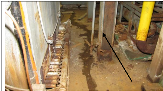
Photograph #9: Basement - active water intrusion
