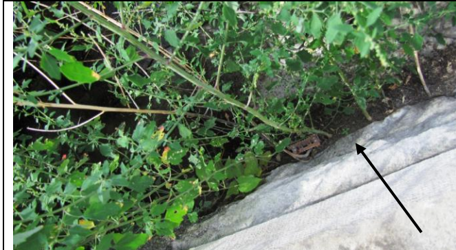
Photograph #7: Heavy vegetation on second floor balcony
