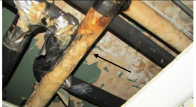
Photograph #18: Above Photograph #17 with visible suspect growth
