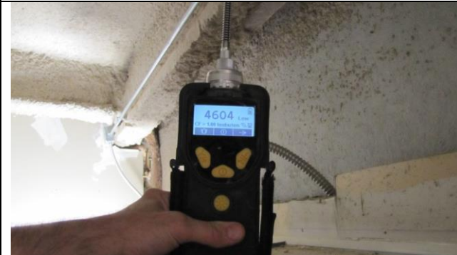
Photograph #6: Elevated PID reading (4.6 ppm) at perimeter
