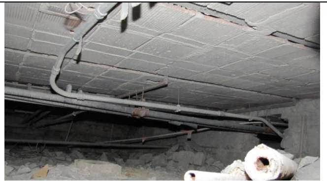
Photograph #6: Debris in crawlspace under west quadrant of building (typical)
