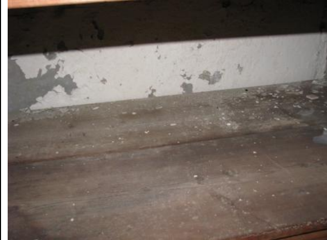
Photograph #49: Basement wipe sample location from shelf (W-36).
