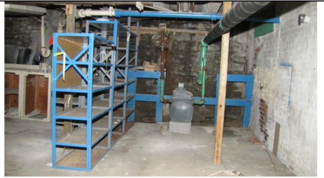
Photograph #8: Basement - active water intrusion
