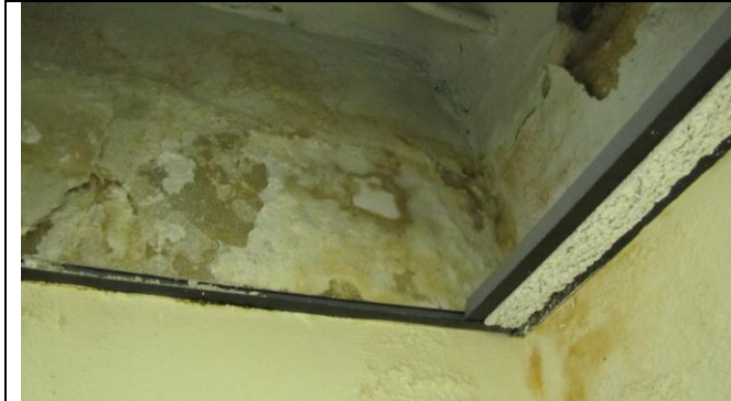
Photograph #11: Visible staining above ceiling tiles in Fallen Heroes Room
