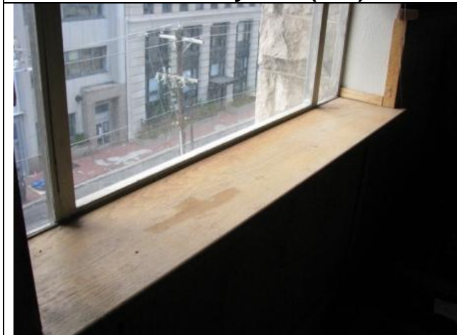
Photograph #21: Wipe sample location 4 th floor window sill (W-7).
