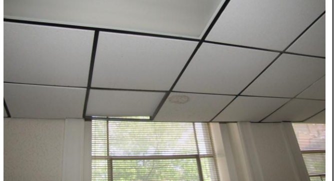
Photograph #20: Room 121 stained ceiling tile northwest wall
