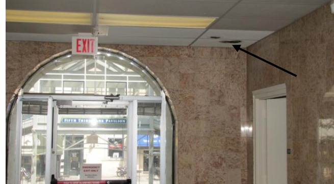
Photograph #19: Northwest entrance of First Floor Hallway with visible growth on ceiling tile
