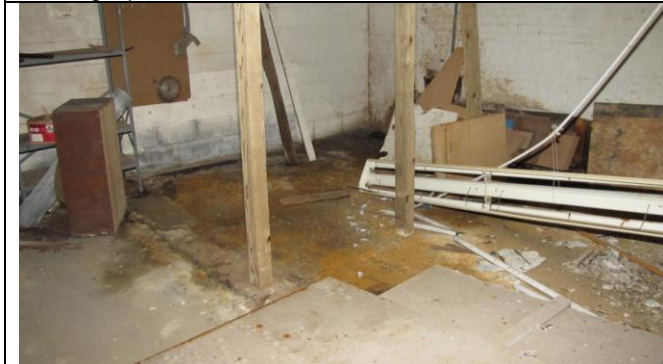
Photograph #13: Basement - active water intrusion
