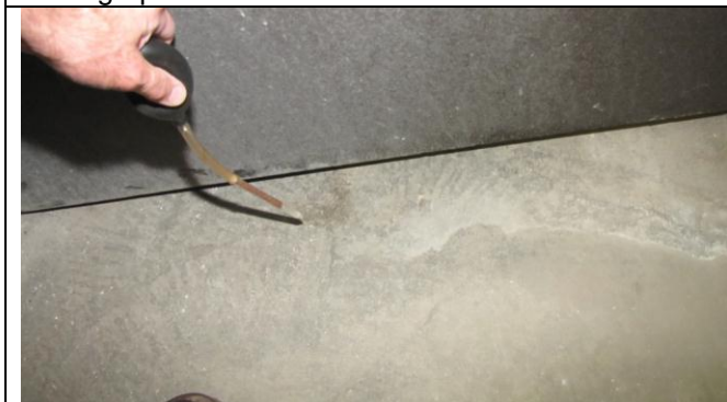
Photograph #15: Penthouse negative with respect to hallway
