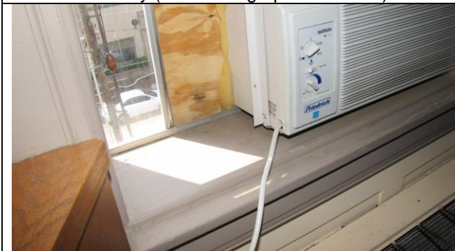
Photograph #31: Another heat pump with poor outward slope (typical)
