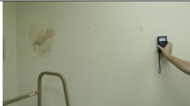
Photograph #13: "Wet" measurement in Fallen Heroes Room inner wall (typical)
