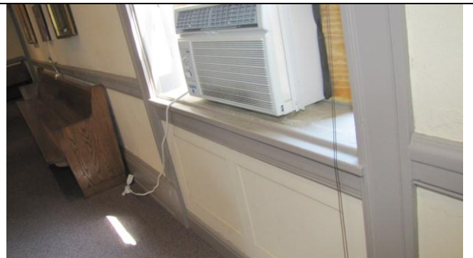
Photograph #30: Room 312 heat pump with poor outward slope
