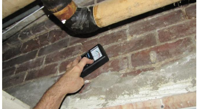
Photograph #24: Above Photograph #17 elevated moisture content
