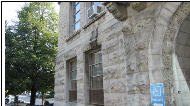
Photograph #5: Under northwest second floor balcony with working heat pump and little evidence of water
