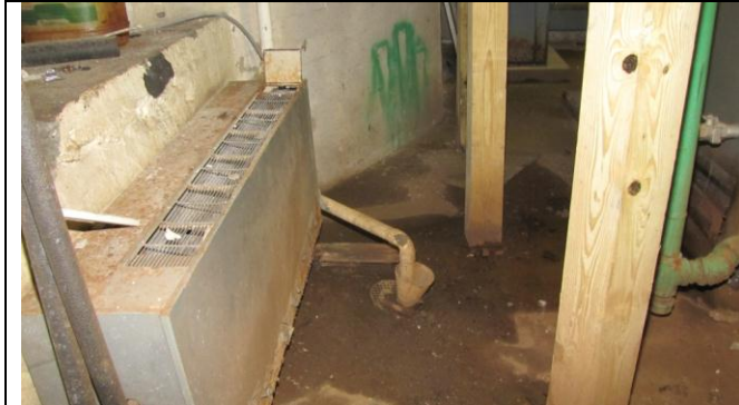
Photograph #11: Basement - active water intrusion
