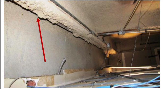
Photograph #10: Gap at perimeter
