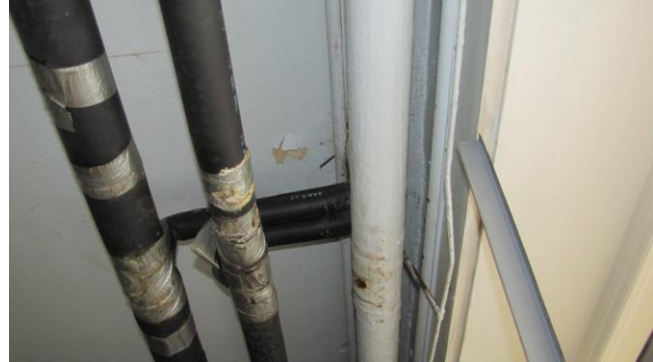
Photograph #21: Air gaps in pipe insulation
