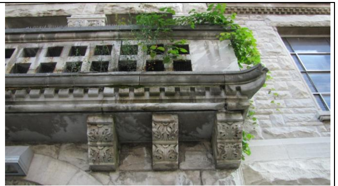
Photograph #6: Under northwest second floor balcony with working heat pump and little evidence of water
