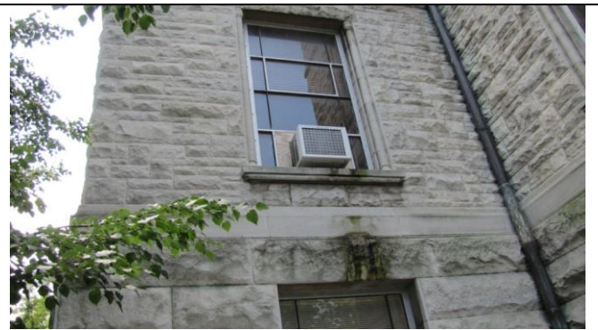
Photograph #34: Condensate from heat pump (southwest wall)
