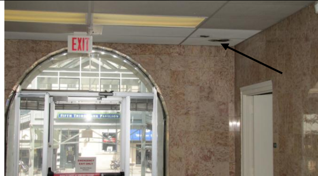
Photograph #17: Northwest entrance of First Floor Hallway with visible growth on ceiling tile
