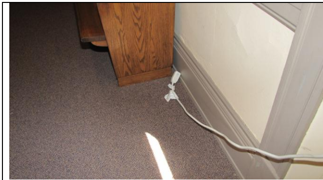
Photograph #33: Extension cord powering heat pump (typical)
