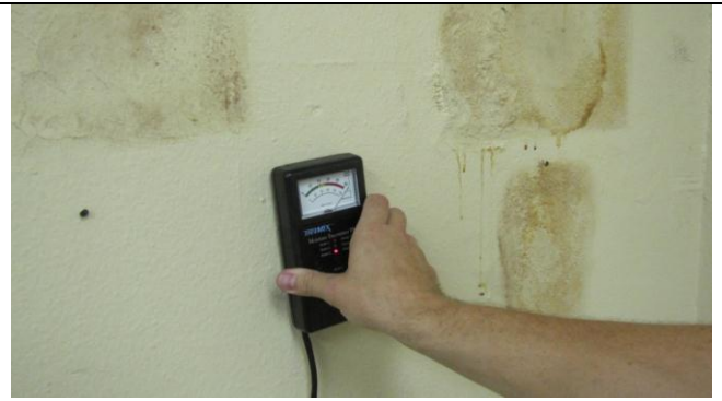
Photograph #14: "Wet" measurement in Fallen Heroes Room outer wall (typical)
