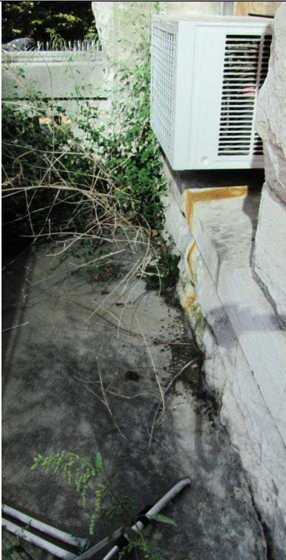
Photograph #3: Northwest second floor balcony with working heat pump
