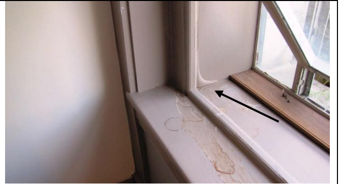
Photograph #8: Water intrusion at second floor balcony window
