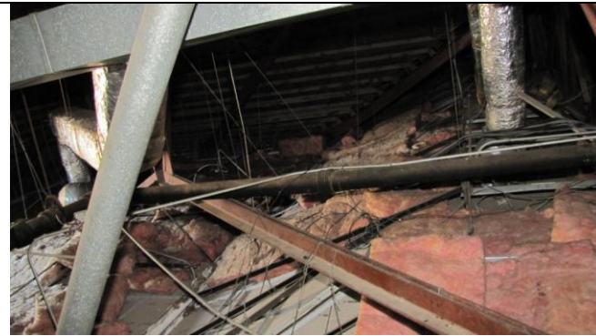
Photograph #17: Attic debris
