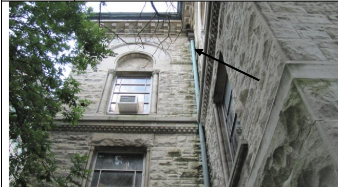
Photograph #27: East corner with overflow from rooftop scupper and poor slope on window-mounted heat pump (Note staining on stone.)
