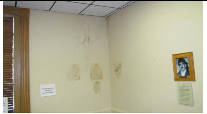
Photograph #2: Northwest wall in Fallen Heroes Memorial Room with visible mold and efflorescence
