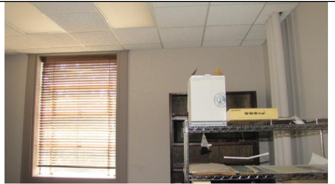
Photograph #26: Third Floor Storage room (east corner) with light musty odor
