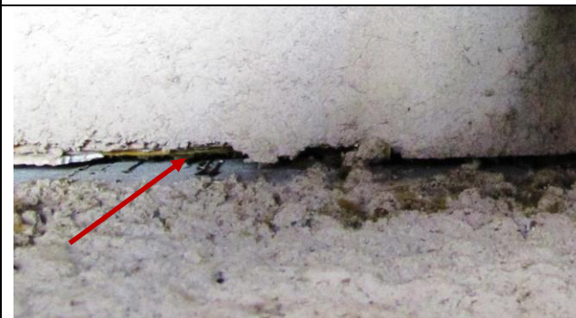
Photograph #8: Drip at perimeter
