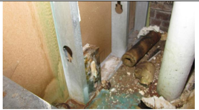
Photograph #4: Debris inside pipe chase and water-stained drywall
