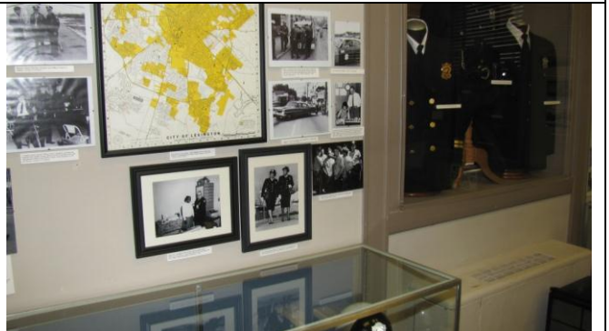
Photograph #22: Public Safety Room (east corner of building) - mold growth reported on backs of pictures
