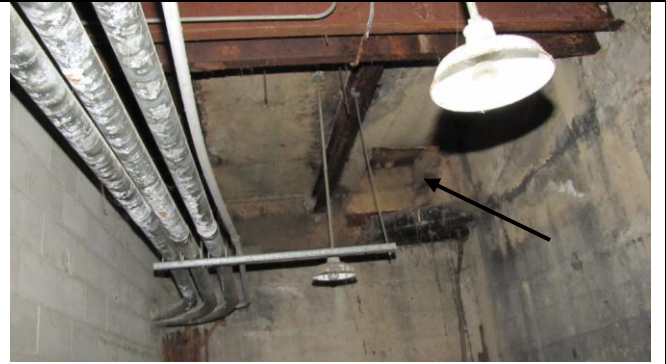
Photograph #12: Basement potential exhaust vent
