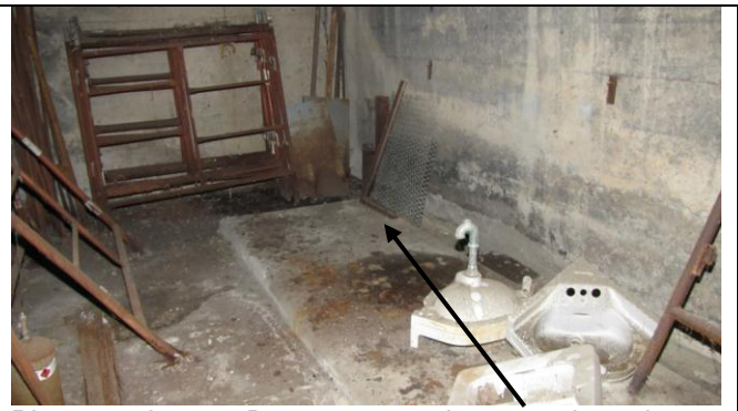
Photograph #10: Basement - active water intrusion
