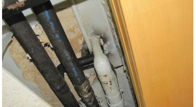
Photograph #16: Above Room 120 stained ceiling tile northwest wall – (Note suspect ACM pipe joint)
