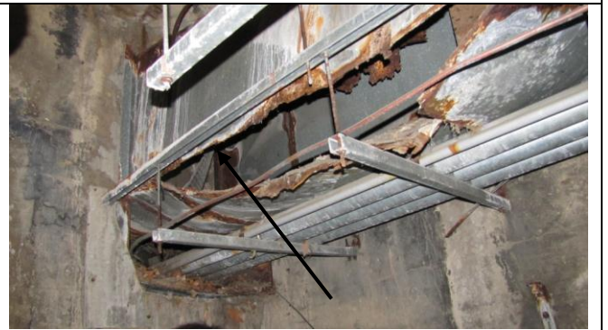
Photograph #10: Basement open grate near sidewalk
