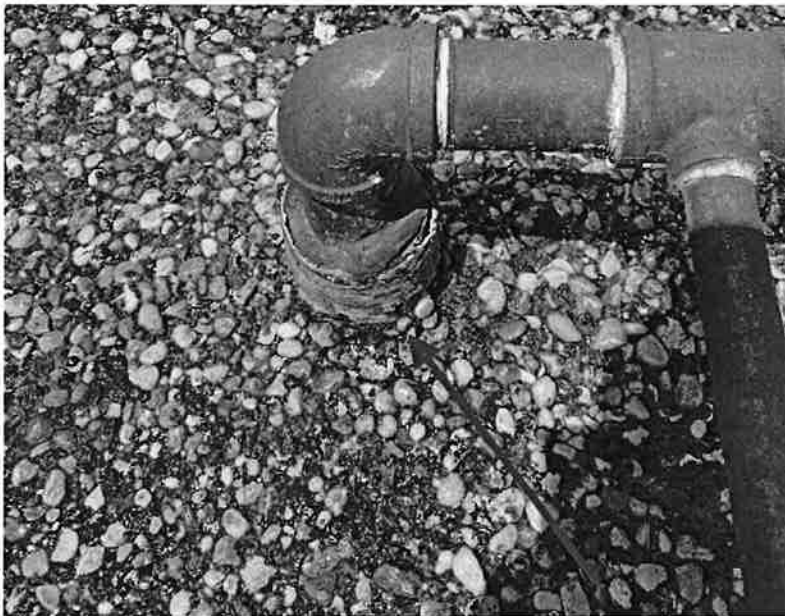
NEEDS TO PROPERLY FLASH AROUND PENETRATIONS OF UNITS
