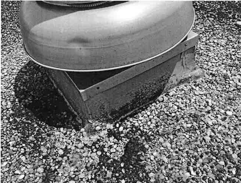
NEEDS TO PROPERLY FLASH AROUND PENETRATIONS OF UNITS
