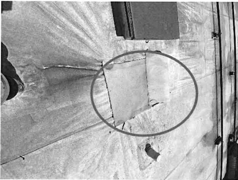
IMPROPER PREVIOUS REPAIRS, PATCH NOT SEAL AND PULLING AWAY FROM ROOF
