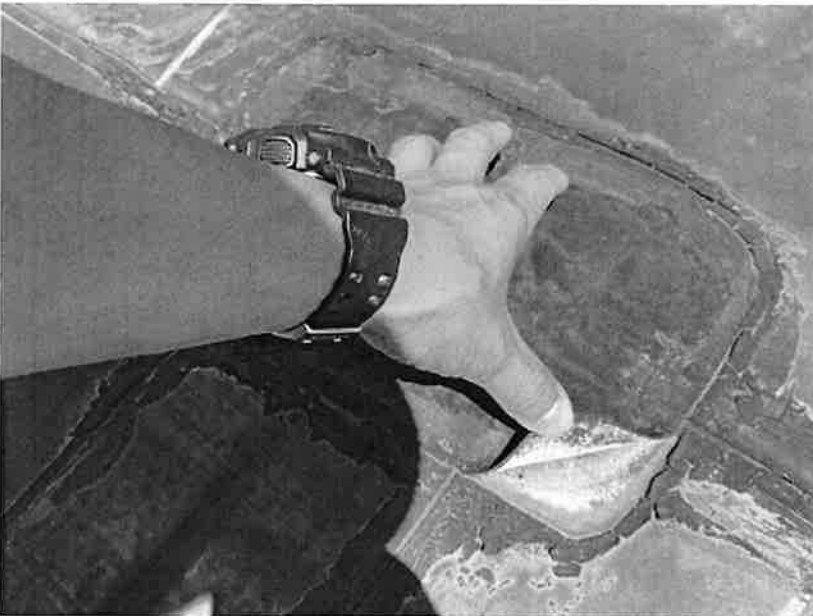
SEAMS NOT SEAL, MAKING IT NO LONGER FUNCTIONAL AND ALLOWS FOR WATER TO LEAK
