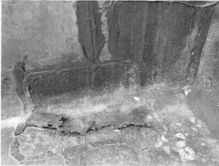
SEAMS NOT SEAL, MAKING IT NO LONGER FUNCTIONAL AND ALLOWS FOR WATER TO LEAK
