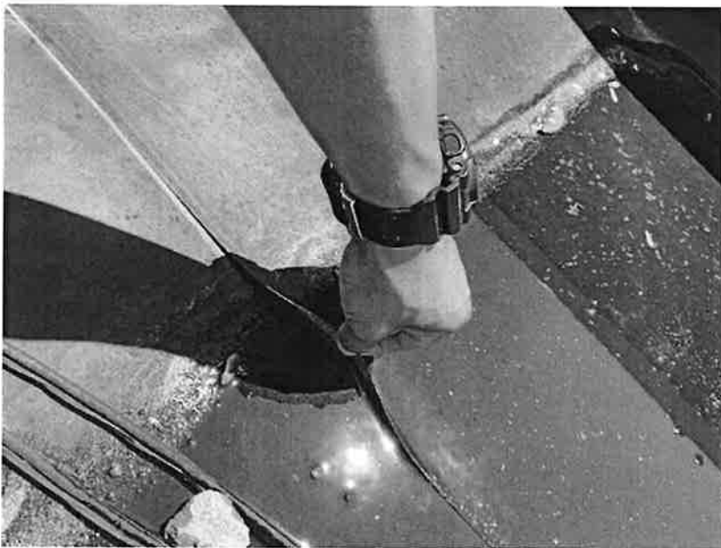
WATER RETENTION ISSUE ALL TRGHOUT THE ROOF AND INADEQUATE SEAL ON EPMD TRANSITIONS ALLOWIG WATER TO PENETRATE AND LEAK
