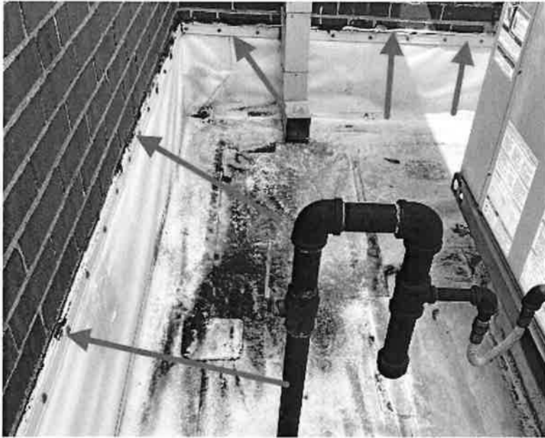
SEALANT NO LONGER FUNTIONAL, NEEDS TO BE RESEALED ALONG WALLS
