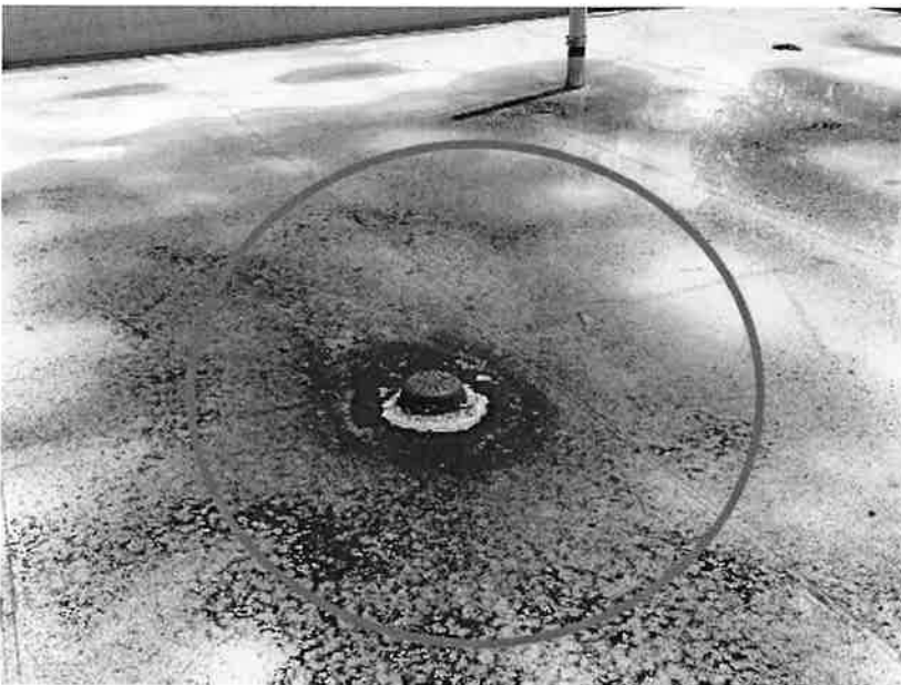
DRAIN SYSTEM CLOGGED UP ON ALL MAIN DRAINS ALLOWING FOR WATER RETENTION ON ROOF
