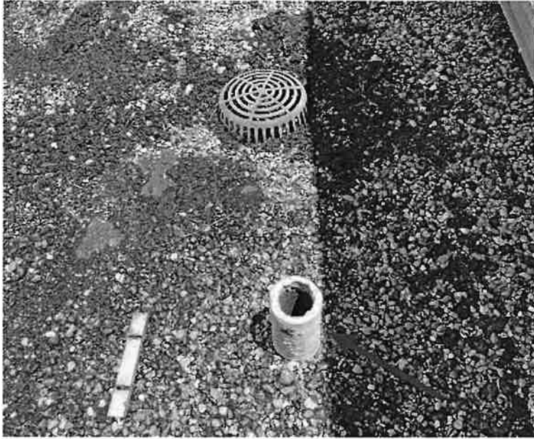
INADEQUATE PIPE FLASHING NEEDS TO BE REPLACED WITH PROPER PIPE JACK FLASHING SYSTEM
