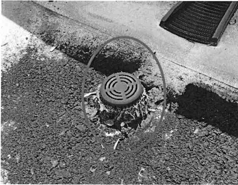
DRAIN SYSTEM CLOGGED UP ON ALL MAIN DRAINS ALLOWING FOR WATER RETENTION ON ROOF
