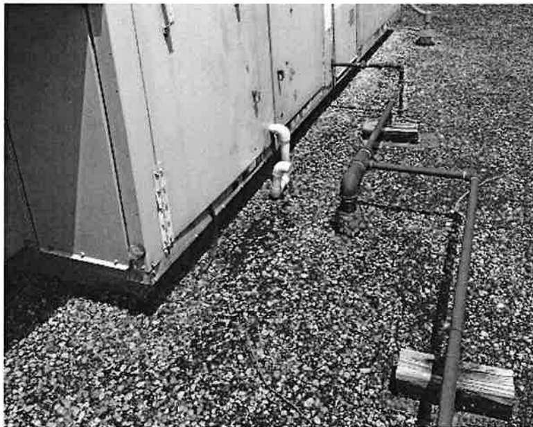
NEEDS TO PROPERLY FLASH AROUND PENETRATIONS OF UNITS
