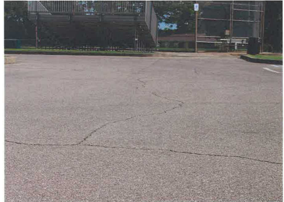
FIGURE #4: examples of single cracks that can be repaired using an asphalt sealer
