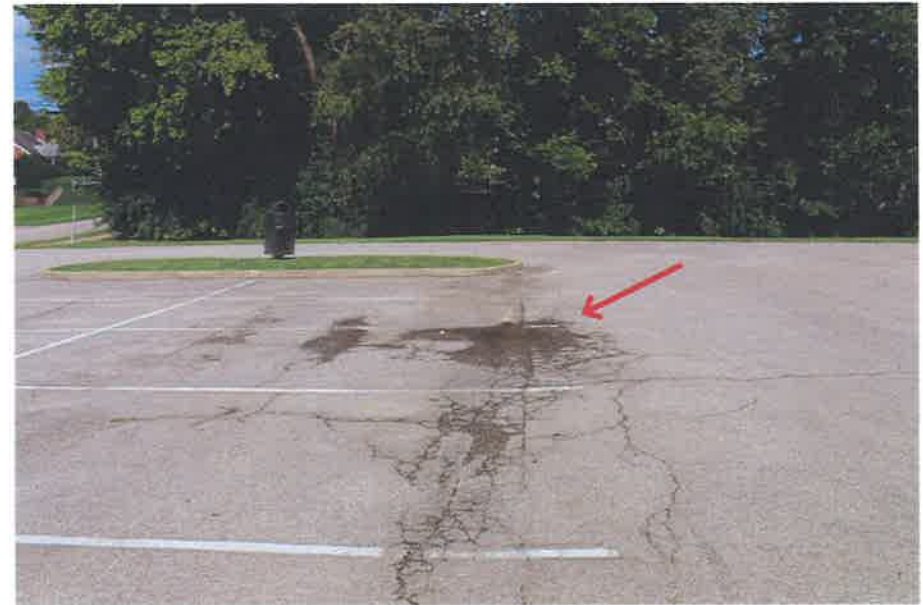
FIGURE #5: examples of multiple cracks that needs further evaluation for more in-depth repairs & early stages of pothole formation (pointed out in red)
