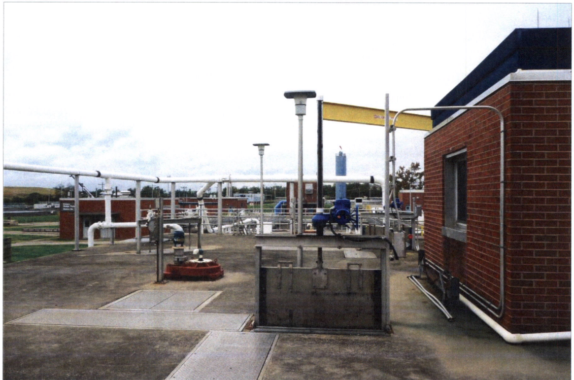
Existing grit removal facilities at Town Branch.
