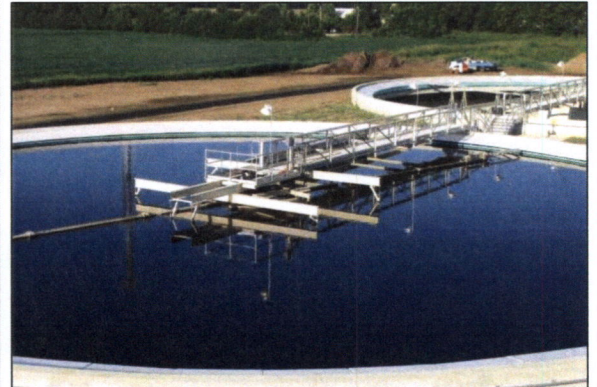
One of four secondary clarifiers.
