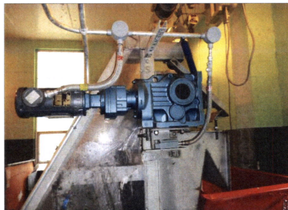
Mechanically cleaned screen installed in existing channel.
