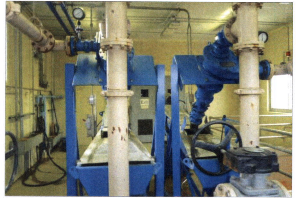
Grit classifier room with limited floor space.
