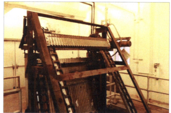
Existing mechanically cleaned coarse screen.
