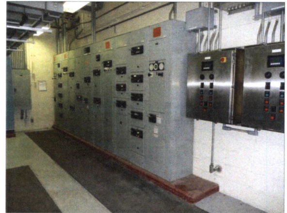
Existing headworks electrical room.
