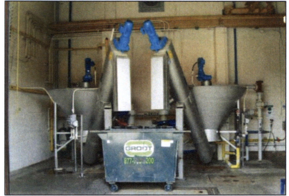
Grit washer units.
