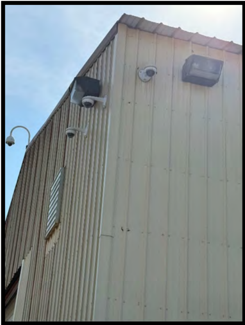
Security Cameras with Lighting on Building
