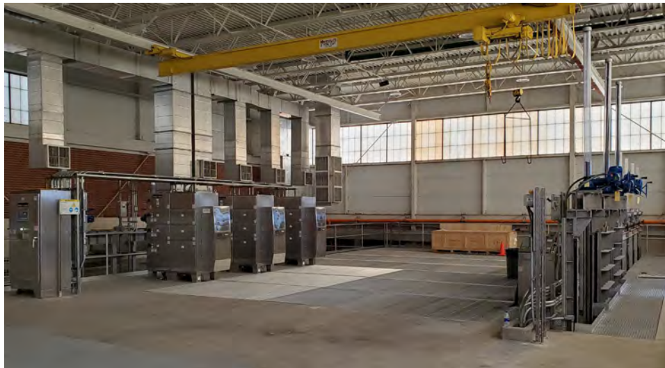
New Trojan UV Disinfection System – Madison Metropolitan Sewerage District.
