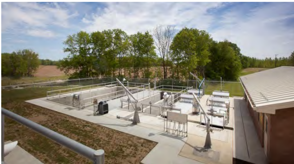
UV Disinfection Process at the CCU WWTF.
