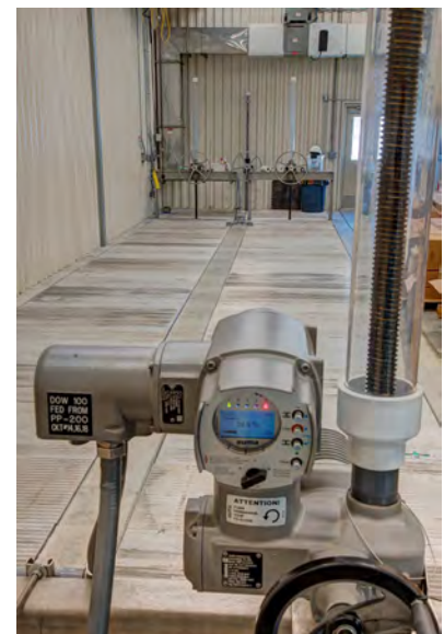
MRP UV Installation with modulating weir level control.
