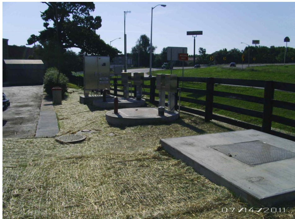
Griffin Gate Pump Station
