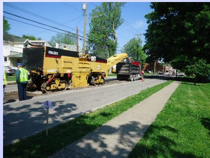
Base failure repair Determined prior to resurfacing
