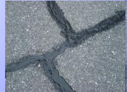
Crack seal 5 years post resurfacing
