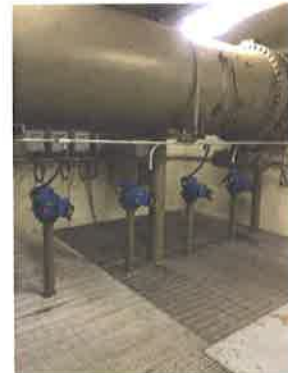
Pump station discharge pipe to aeration influent.
