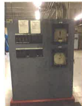
Existing motor panel.
