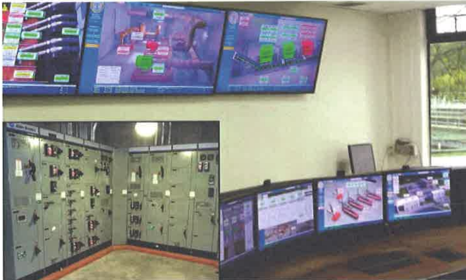
SCADA control room allows the plant operator to control and monitor WWTP operation.
