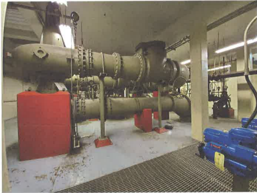
GENERAL PHOTO OF THE AREA AND PIPING
