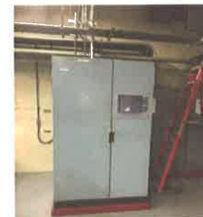
DCU upgraded in recent SCADA replacement project.
