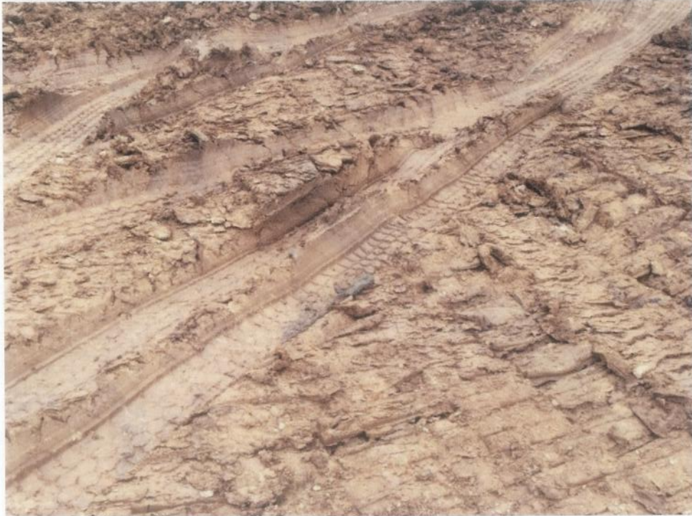
Photo 5: View Of Ruts In The Cul-De-Sac Area
