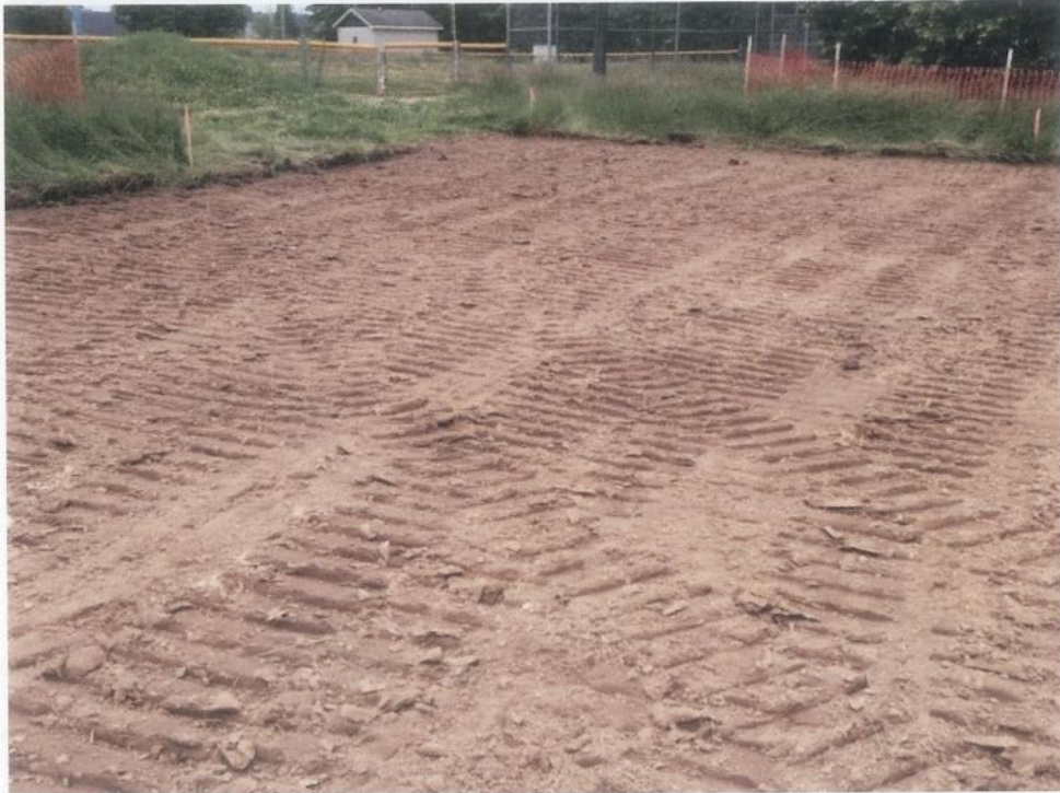
Photo 7: View Of Basketball Court Cut To Grade With Mixture Of Top Soil And Clay
