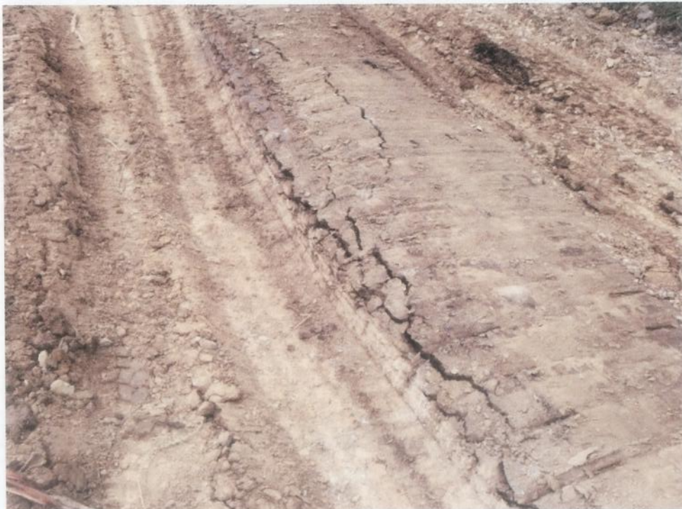
Photo 6: View Of Ruts On Section Of Roadway
