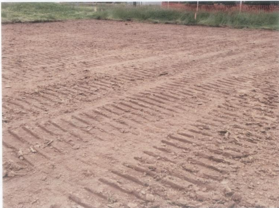
Photo 8: View Of Basketball Court Cut To Grade With Mixture Of Top Soil And Clay
