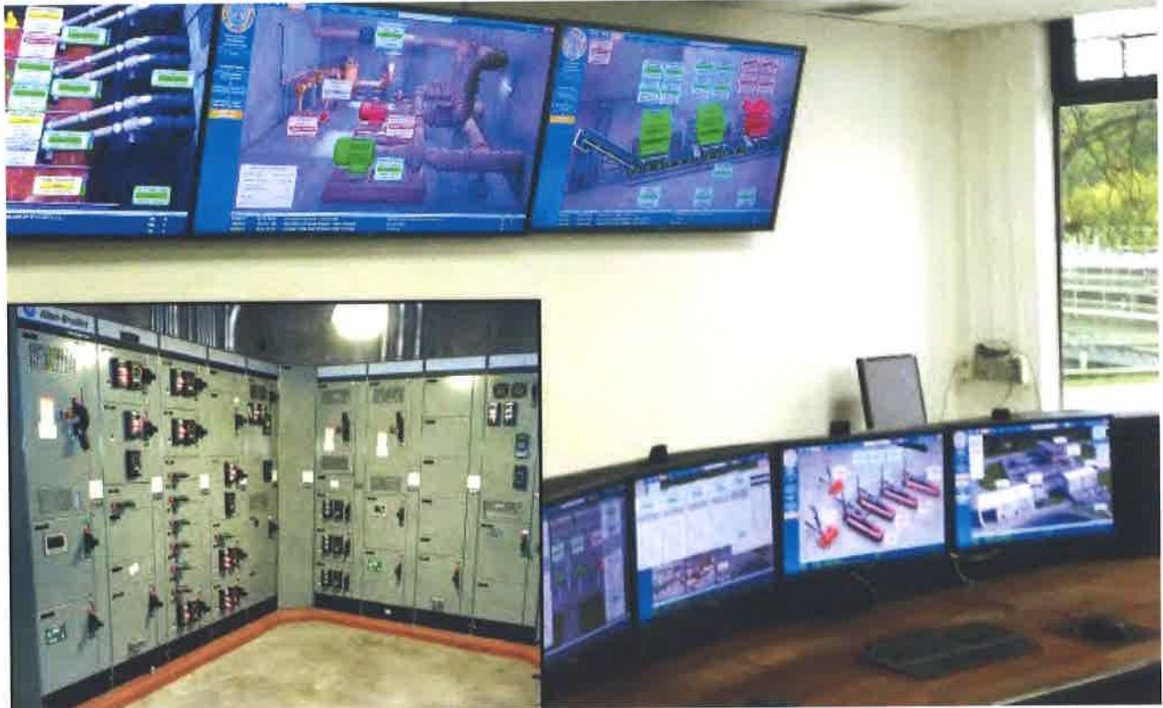
SCADA control room allows the plant operator to control and monitor WWTP operation.
