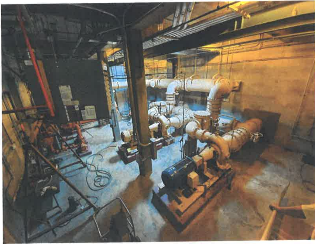
BUILDING #12 – 2 RAS PUMPS
