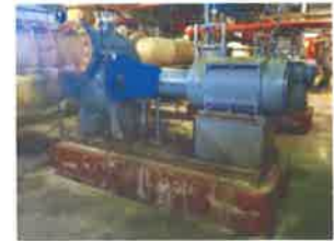
RAS Pump Nitrification Gallery.
