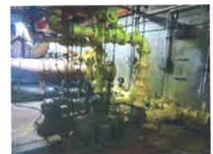
WAS/Scum Pumps 1-3 Nitrification Gallery.
