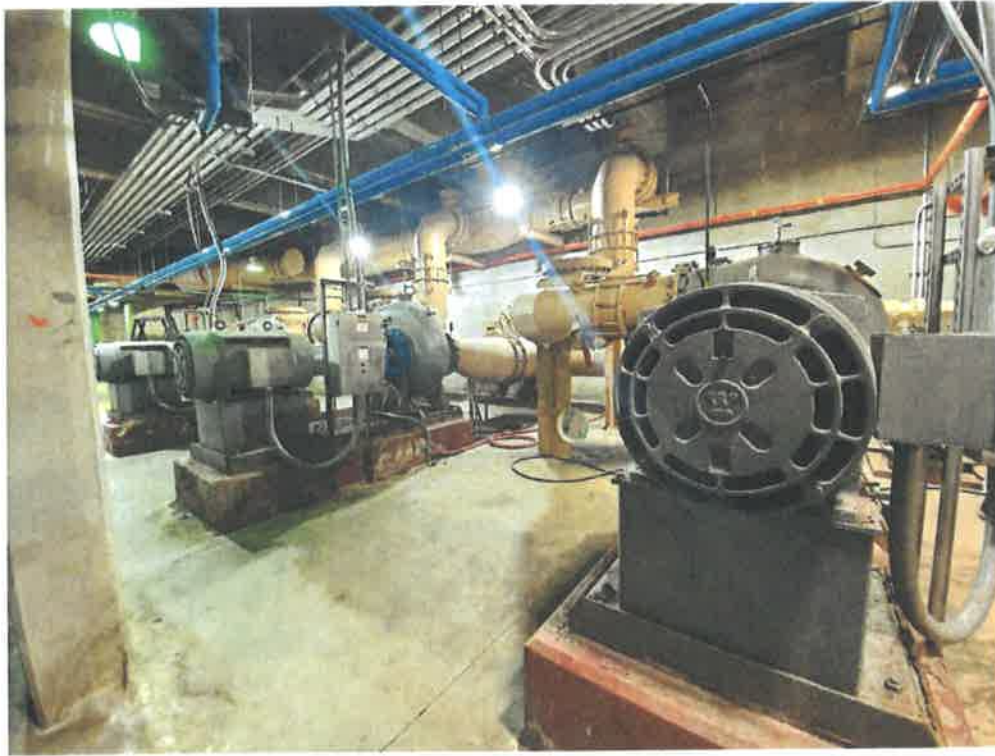
BUILDING #11 – 3 RAS PUMPS
