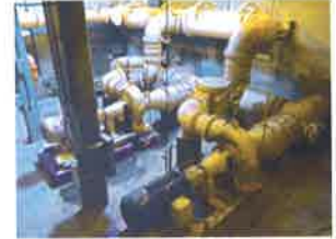
RAS Pumps 445 Nitrification Return Sludge Pump Station.
