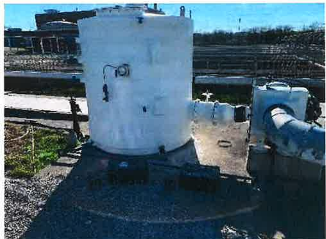
Odor Control System Testing Town Branch WWTP
