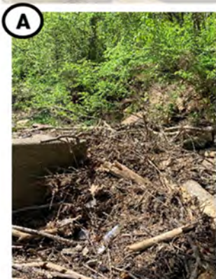
A Erosion has disconnected the low head dam from the stream's right descending bank.
