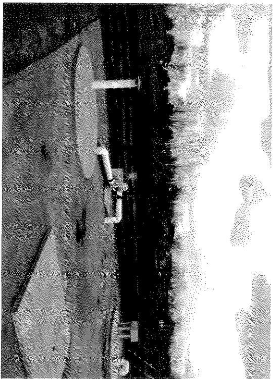
Blackford Property Pump Station
