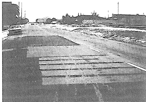
Reclamite was used as a construction seal on the dry areas of the pavement.
