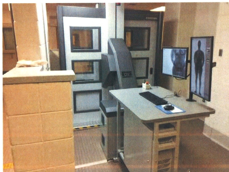
CONPASS DV with Optional XSC Safety Cabin (Fairfax County Jail – VA)
