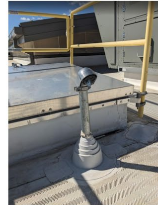
Electrical weatherhead "e"
